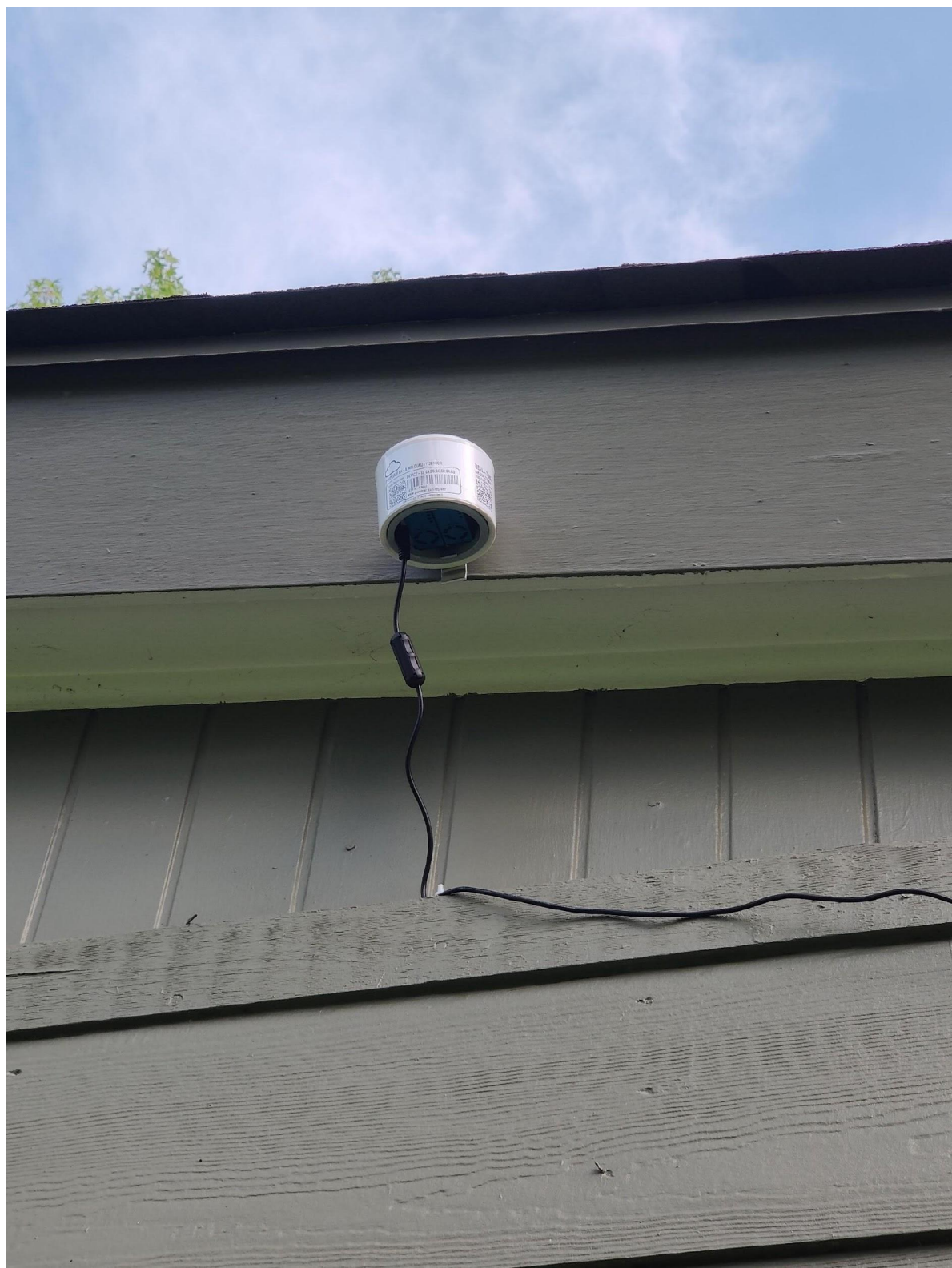
Installed Purple Air Monitor
